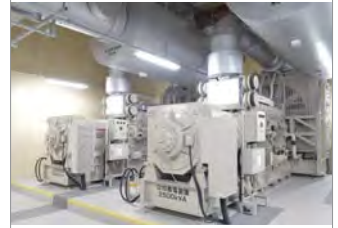
Emergency electric generator
