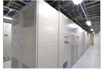
Uninterruptible power supply (UPS)
