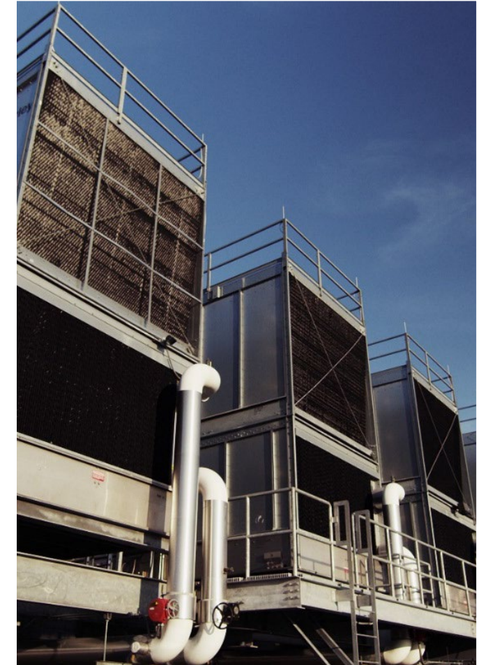
Data Center Cooling Towers
